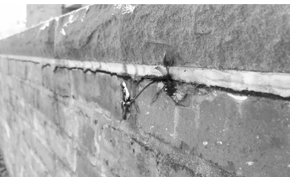
A dandelion in a brick wall at MASS MoCA, November 2016
